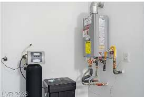
Essential utilities showcase a modern tankless water heater and water softener system.
